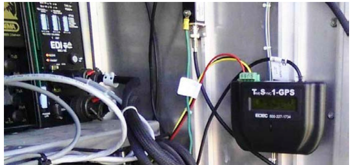
TimeSync1-GPS mounted inside cabinet using DIN Rail.
